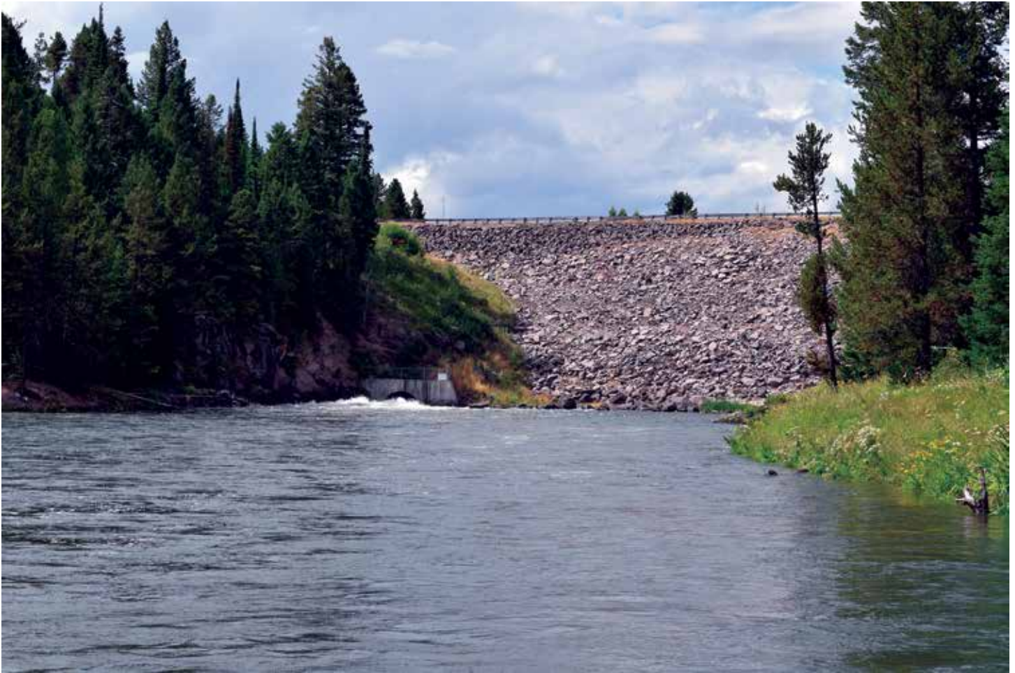
Figure 2. Island Park Dam (background) and the Henry's Fork River (foreground), showing the USBR hypolimnetic outlet on the lower-left part of the dam. Picture was taken on July 22, 2015, during peak irrigation delivery.
